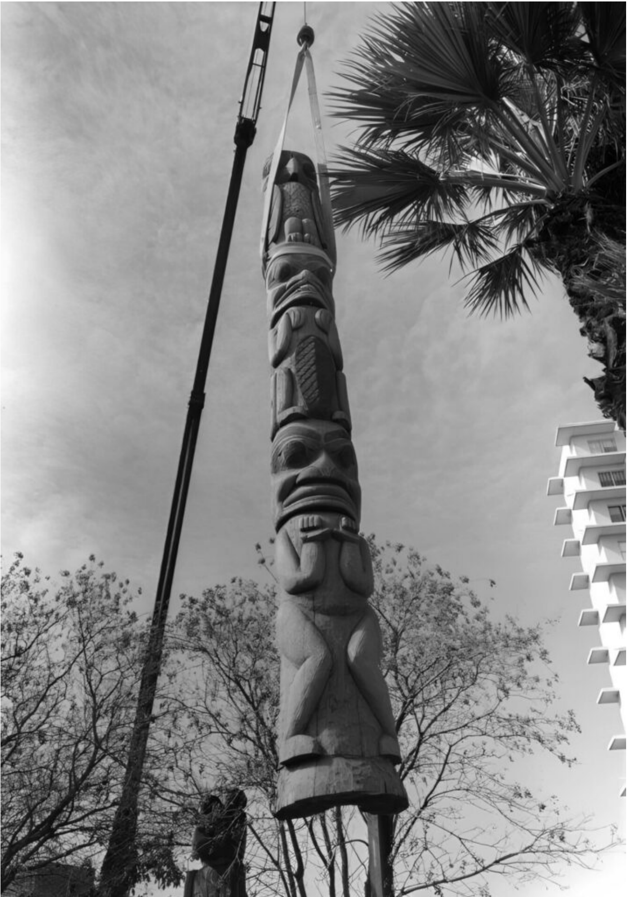
The Friendship Totem is lifted by a crane for installation on the Heard Museum grounds in 1976.
